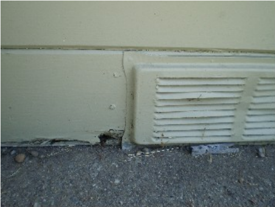
Damage to wall in lower rear bedroom, near vent. Treat and repair.
