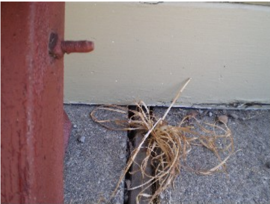
Gap under wall in rear of kitchen. Repair.
